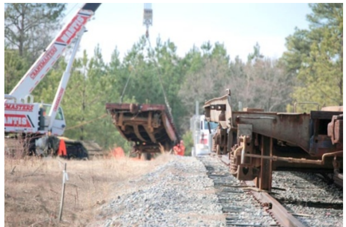
Fort Lee Photo/Rhonda Seward A crane moves railcars onto a rail spur at Fort Lee on Jan. 11 for movement to their final destination at the Army Transportation School multi-mode load training site.
